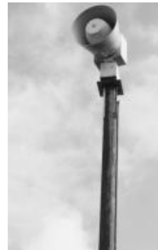
NEW SIRENS UP - Five new weather warning sirens have been installed in Rankin County, including the Patrick Farms area, the Robinhood and Star communities, Buckingham subdivision near the Reservoir, and along Gulde-Shiloh Road near Brandon. The county received FEMA funding for the purchase, and officials have applied for an additional round of funding.
